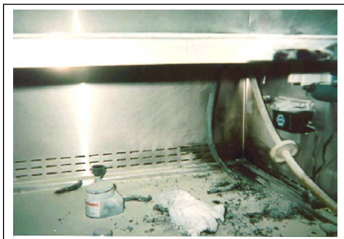
A fire inside a BSC occurred when the gas rubber hose connected to a Touch-O-Matic Bunsen burner melted and gas in the hose ignited. Brookhaven National Laboratory, Lessons Learned 2002-CHBNL-MED-0003 (July 23, 2007).
